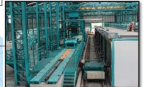
Individual curing carrousel with Vibration table Thailand Bangkok City Metro
